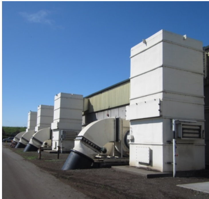
Figure 2-3: Compost Building Exhaust Fans
