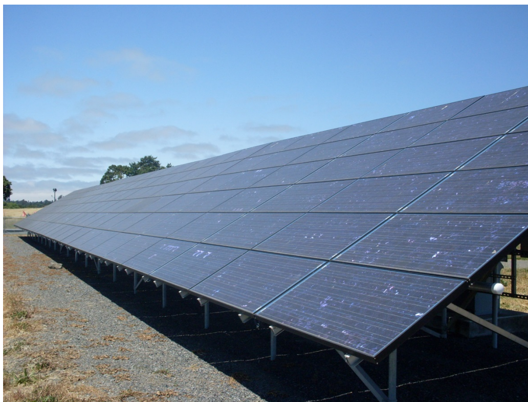
Figure B-1: Fixed Tilt System Installed at Laguna Treatment Plant
