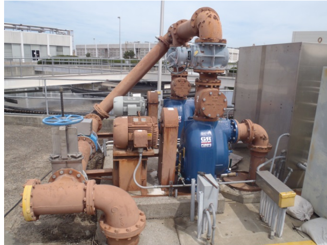
Figure 1-9: RAS Pumps Adjacent to the Clarifier
