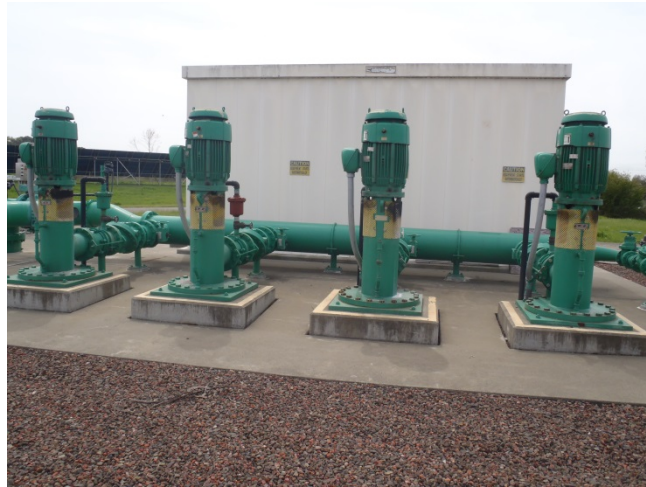
Figure 1-6: Recycled Water (3W) Booster Pumps
