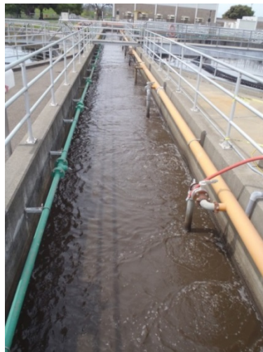
Figure 1-7: Mixed Liquor Channel with Aeration
