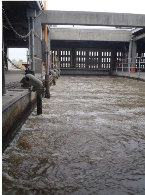
Figure 1-11: Grit Tank with Aeration
