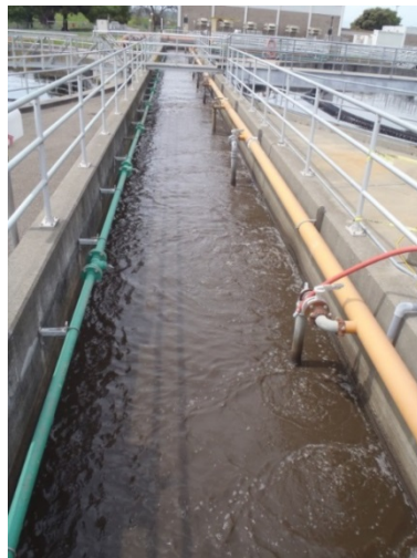
Figure 1-7: Mixed Liquor Channel with Aeration
