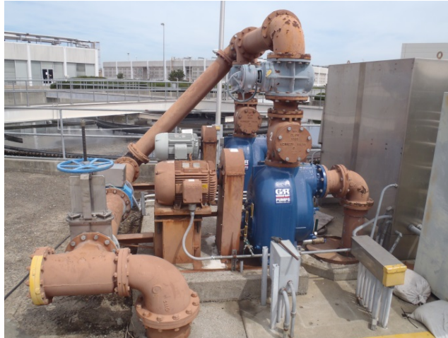
Figure 1-9: RAS Pumps Adjacent to the Clarifier
