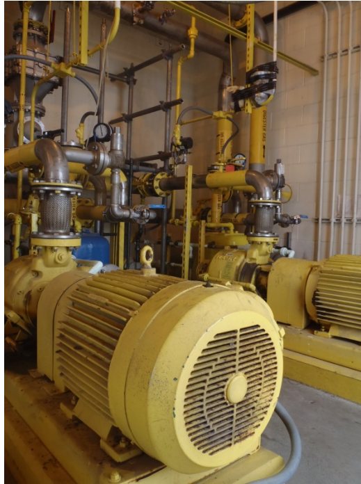
Figure 1-10: Digester Gas Mixing Pumps
