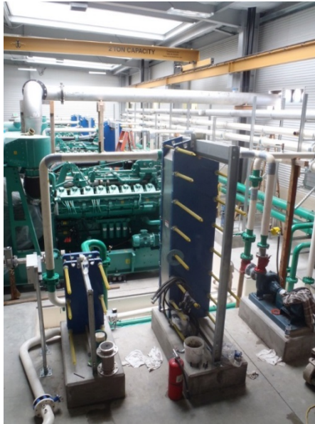
Figure 1-8: Overview of the CHP Facility
