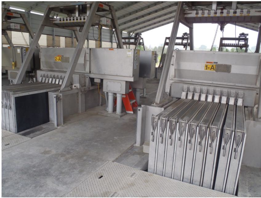
Figure 1-4: UV Disinfection Equipment
