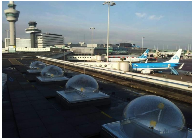
Figure 11: Sun-tracking Skylights with Mirrors
