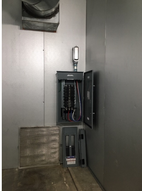
Figure 12: Electrical modifications in the BSRL large environmental chamber
