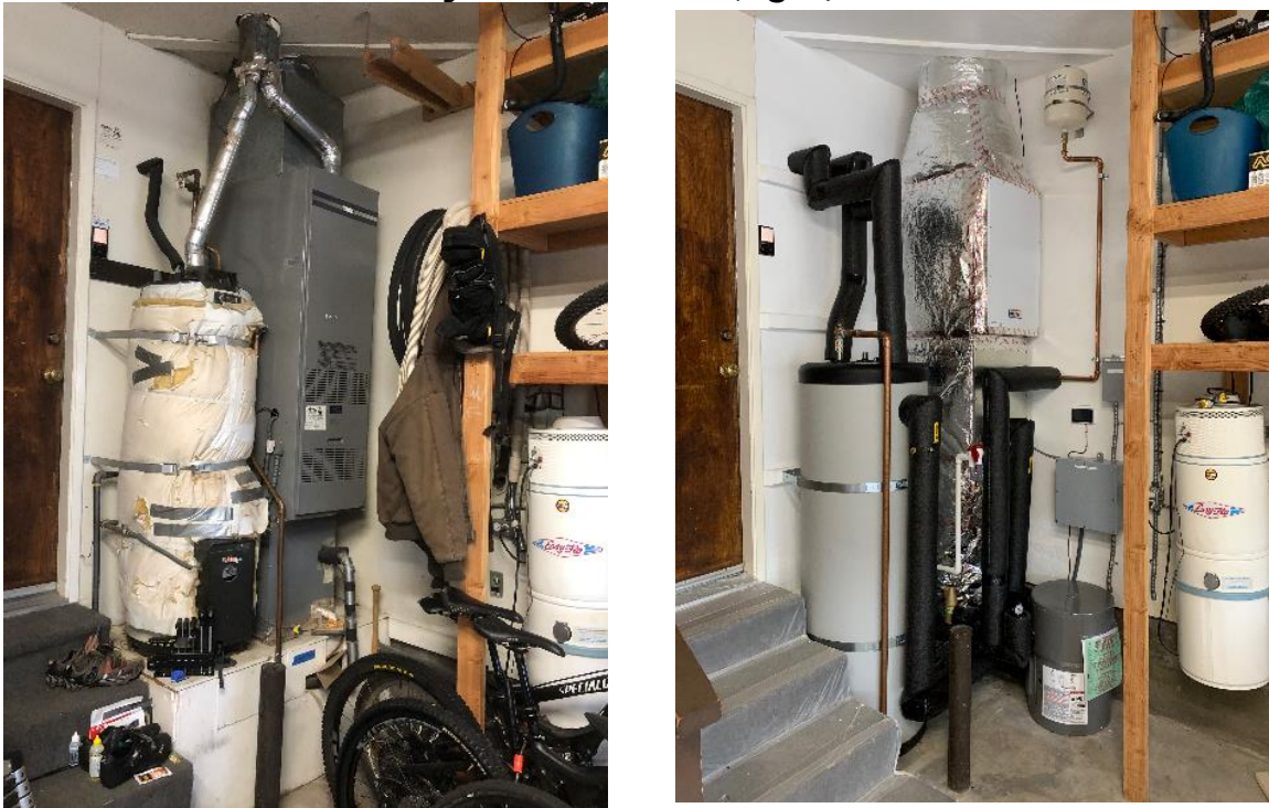
Figure 27 - Existing gas water heater, gas furnace, and air handling unit (left). New indirect water heater tank, expansion and backup tanks, air handling unit and hydronic fan coil (right).
