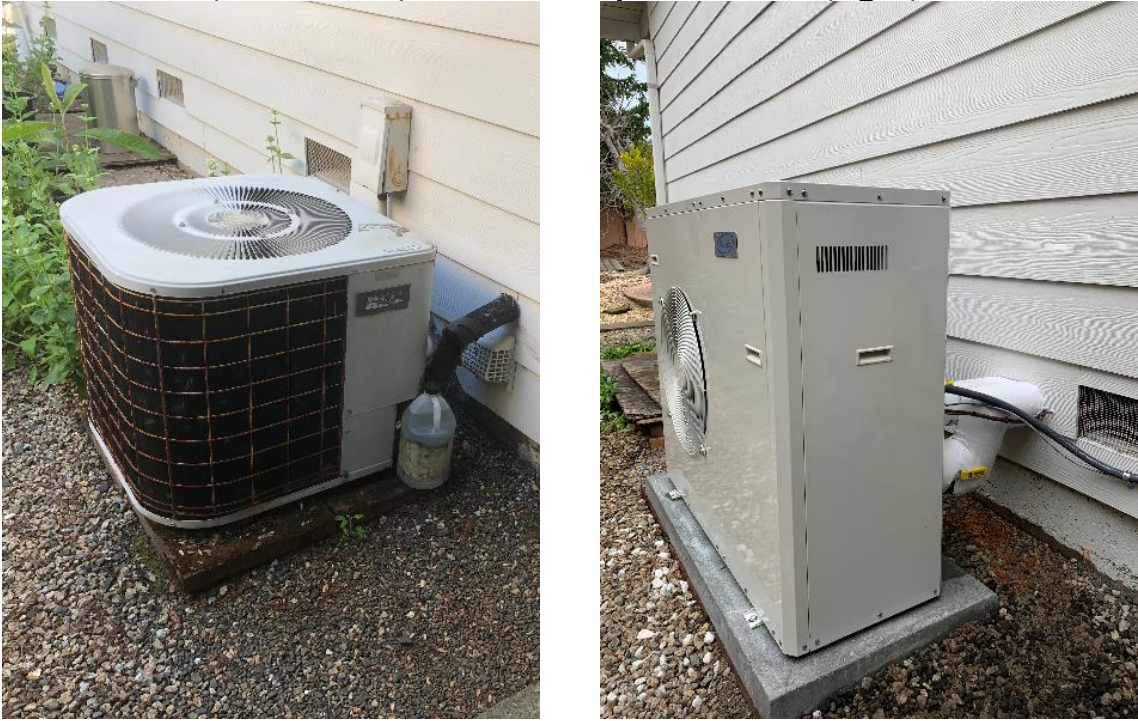
Figure 26 - Existing condensing unit prior to retrofit measure (left), and AWHP (Citrix CX34) as installed post retrofit (right).
