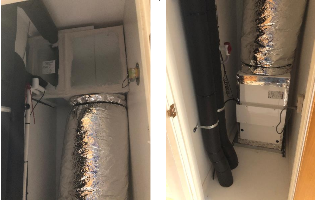
Figure 30 - Closet holding the air handling unit (bottom), and the hydronic fan coil (top).
