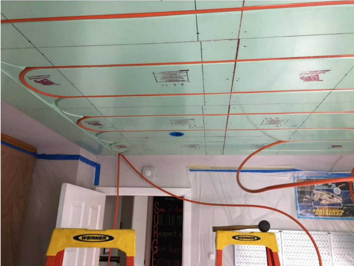
Figure 17 - PEX pipes were mounted inside the precut channels of the radiant panels.
