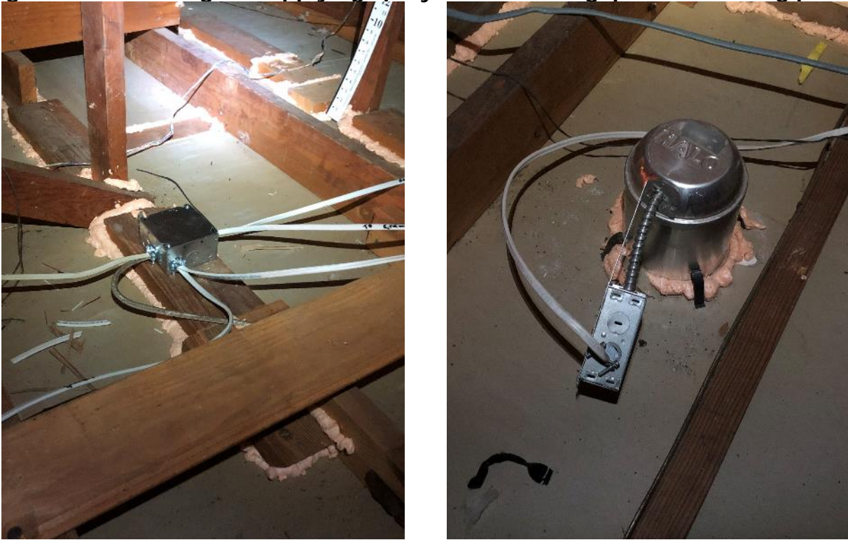
Figure 31 - Caulking and applying spray foam to seal gaps in the ceiling plane.
