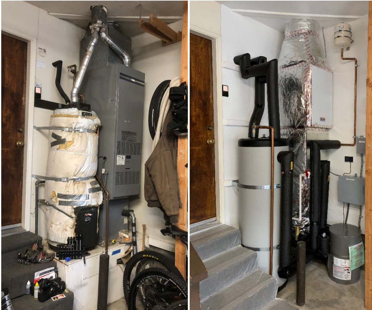
Figure 4. Left: Old equipment which included a gas water heater and furnace. Right: Replacement equipment which includes an indirect DHW tank, hydronic air handler, and buffer tank.
