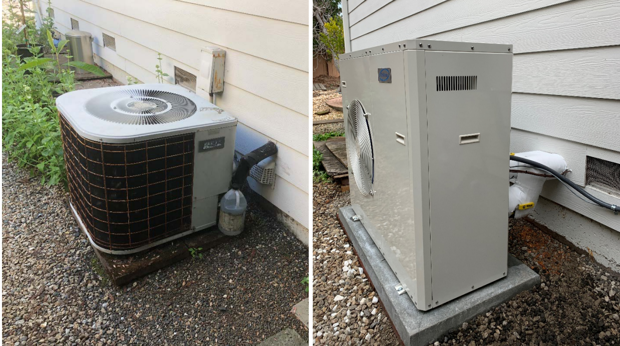
Figure 3. Left: Old outdoor unit. Right: New outdoor unit, installed in approximately the same location as old unit (moved back a bit for clearances).
