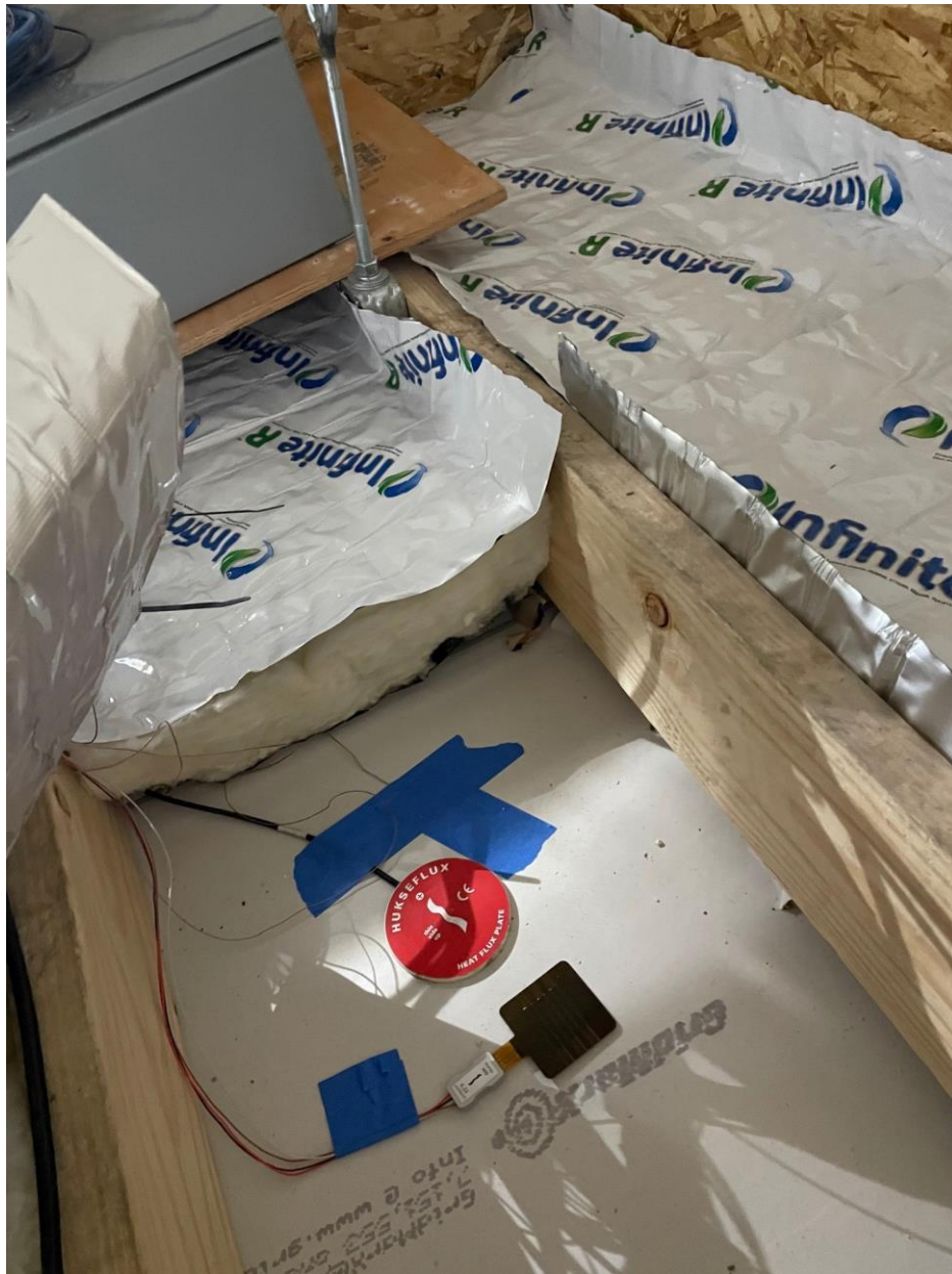
Figure 10: Heat flux sensors installed under insulation during lab testing
