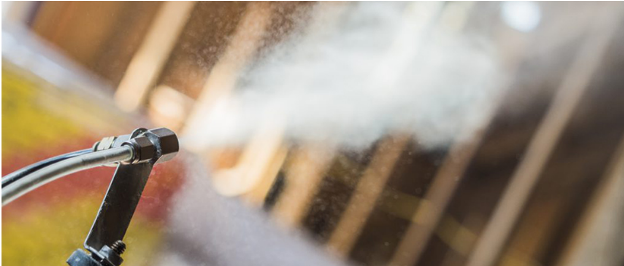
Figure 6: Aerosolized Sealant Released into the Interior of a Building
