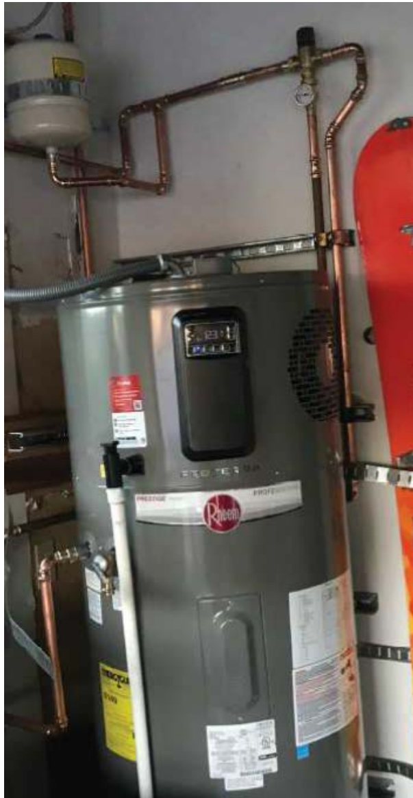
Figure 2: Installed GIHPWH with Thermostatic Mixing Valve
