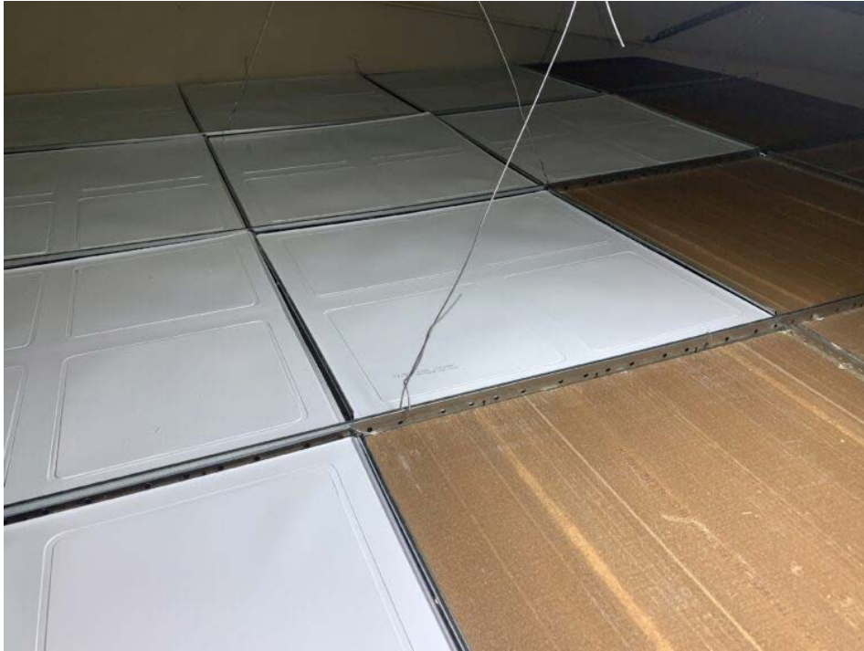
Figure 10: Templok PCM Tiles in Drop Ceiling
